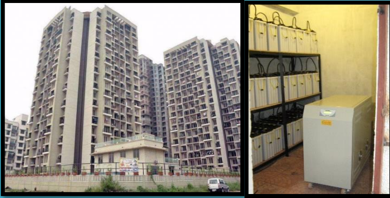
50KVA LIFT UPS at ARIHANT ABHILASHA, Navi Mumbai
