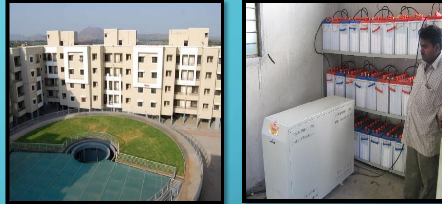
75KVA LIFT UPS for Township at ADARSHA VISHWA, Satara
